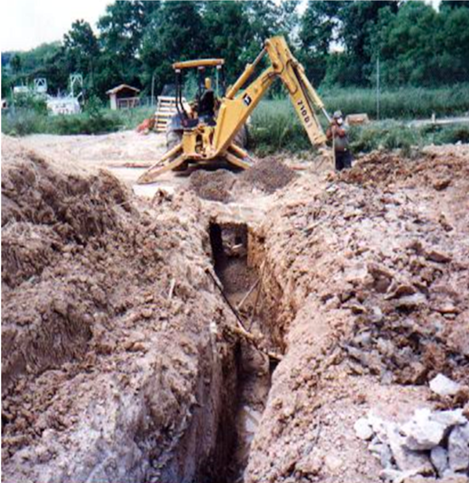
Photo of deep excavation without protective system
