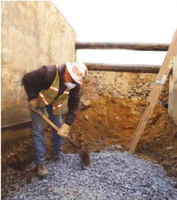
Photo showing the allowable gap between the bottom of the trench box and trench bottom
