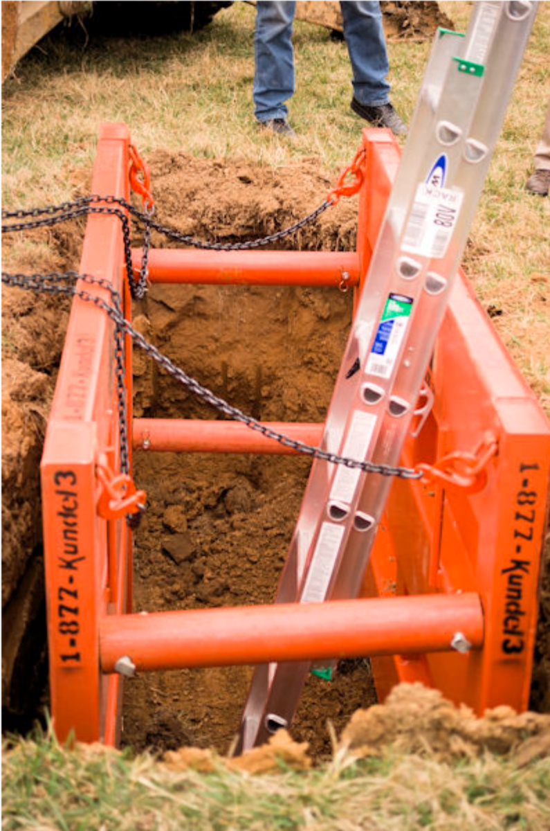
Photo showing a trench box without soil backfilled against the sides of the box
